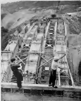
Located four kilometers from Catia, Bridge No. 1 is 392 meters long and 70 meters above the Tacagua ravine. Two workman are shown fastening steel reinforcement wires before pouring concrete at No. 1.
